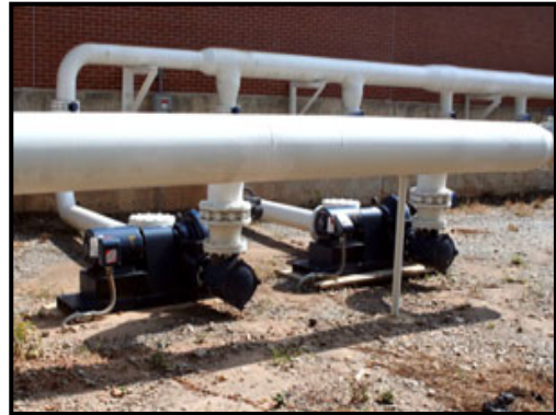
Water Pumps Fueling the A/C Units
