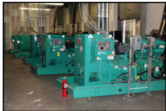
Backup Power Generators
