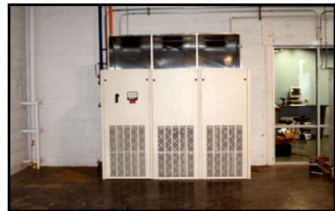
An A/C Unit Cooling the Server Area
